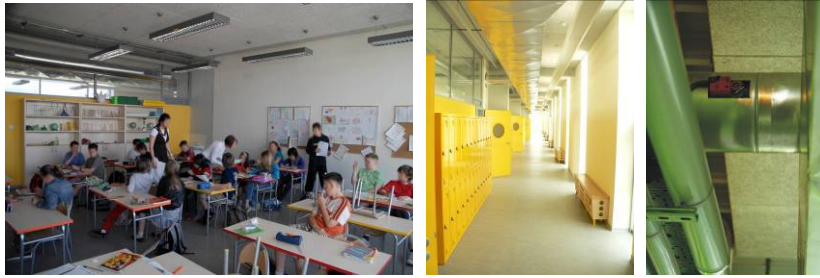
Fig 1.3 a) Classroom with MV ducts visible, b) Corridor with MV ducts visible, c) Location of the control gear for MV at ceiling high
